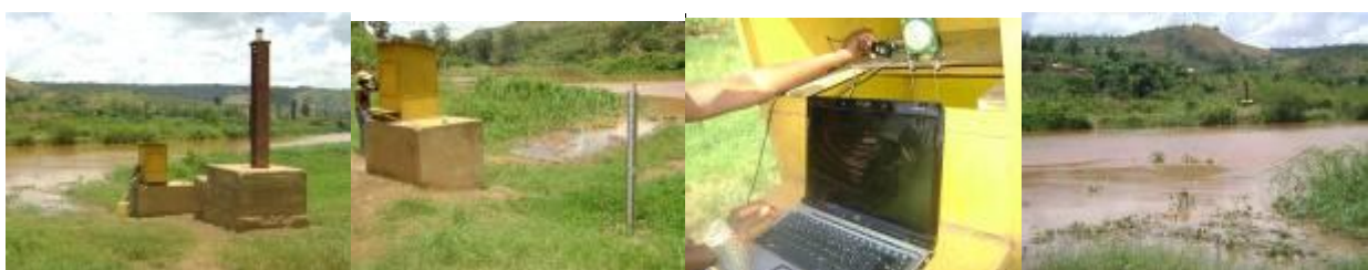
Figure 3.3: Gauging station installed at Rusumo for water level measurement of Kagera River
