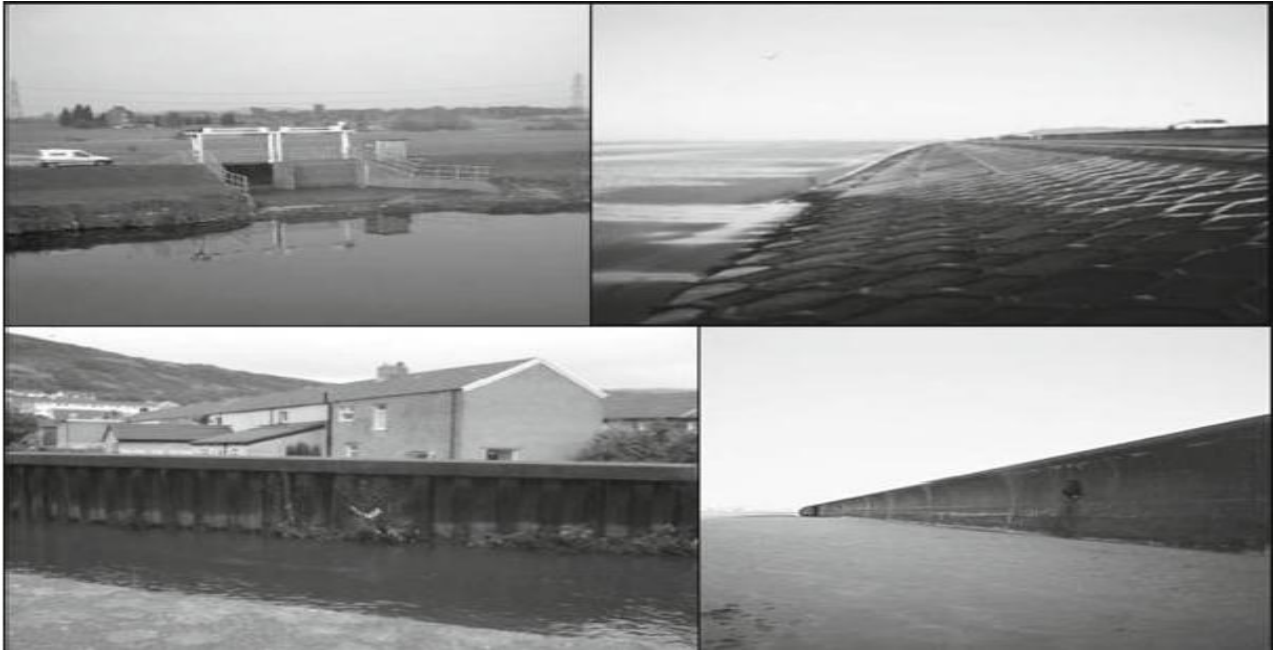
Fig. Examples of river and coastal flood defences and a flood gate for wash land drainage
