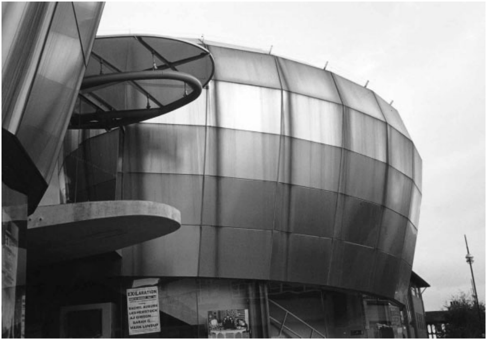
Figure 13.2 Stainless steel cladding may have appeared to be contextually appropriate on the former National Centre for Popular Music in Sheffield but was it the best material to use in terms of building form and location? The cladding was stained and streaked with dirt within a few months of the building being completed.
